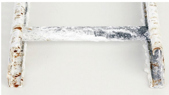
Traditionally hot-dip galvanized cable ladder.
