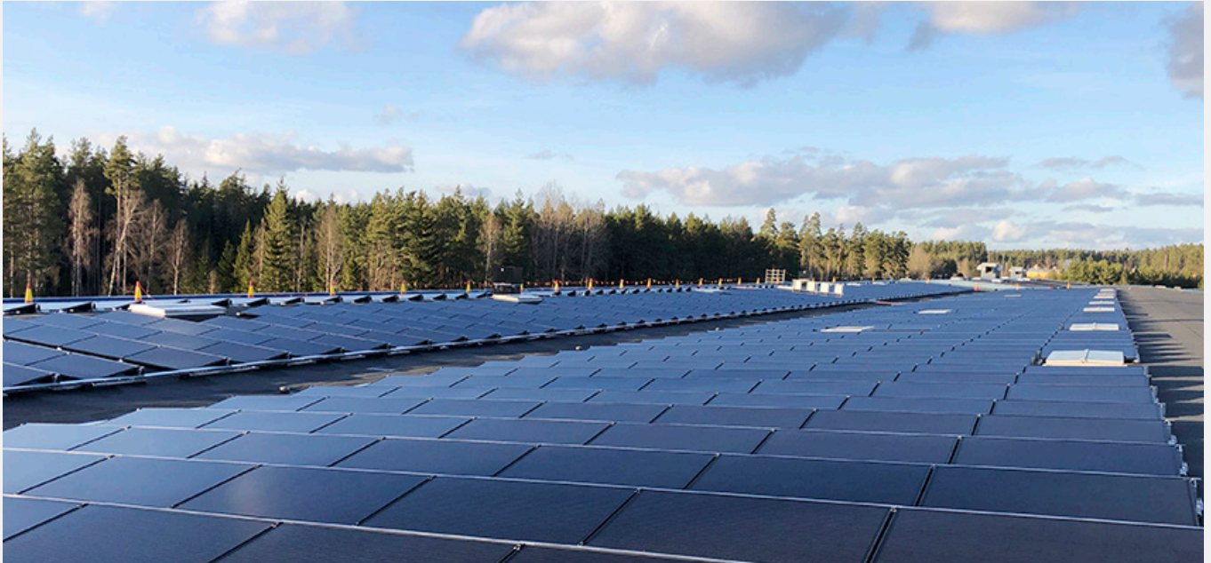
MP bolagen's factory on Barkvägen in Ekenässjön, where the roof is now utilised for environment-friendly electricity production.
